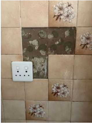
Ref #5.6 - Missing tiles
