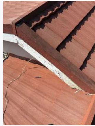
Ref #7.5 - Damaged fascia
