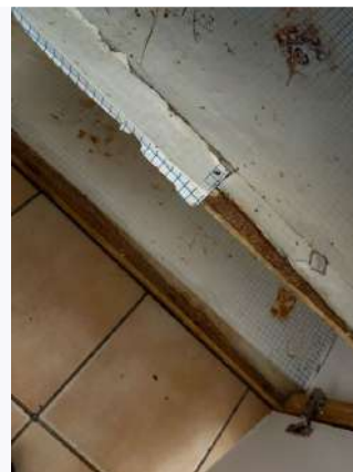
Ref #5.2 - Significant damage to cupboards
