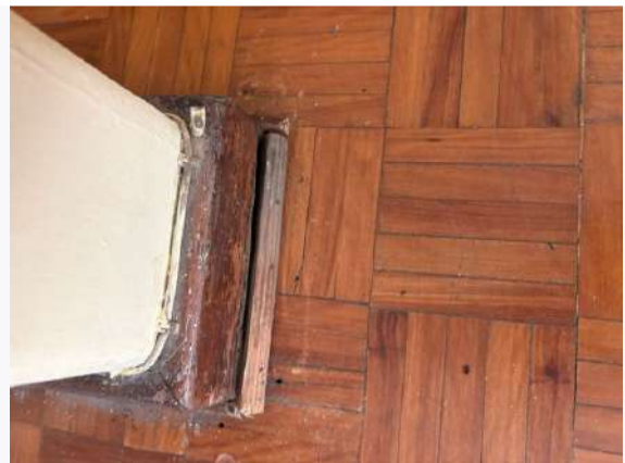
Ref #3.3 - Lounge floor with wood damage
