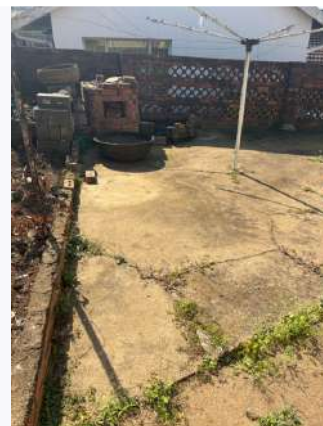
Ref #12.1 - Evidence of water ponding/Ground subsiding
