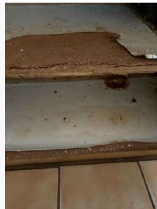
Ref #5.2 - Significant damage to cupboards
