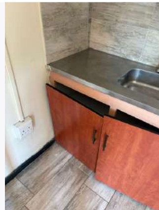
Ref #13.1 - Damaged doors
