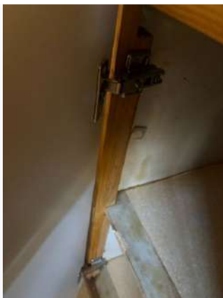
Ref #5.2 - Significant damage to cupboards
