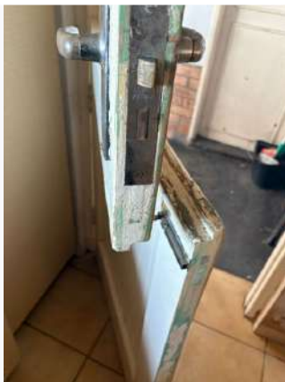
Ref #5.1 - Flaking paint
