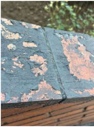
Ref #11.5 - Damaged capping
