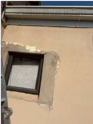
Ref #13.3 - Crack in wall
