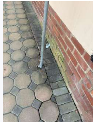
Ref #12.3 - Paving subsided
