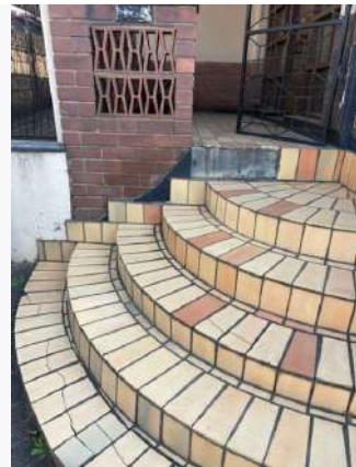
Ref #11.3 - Damaged tiles
