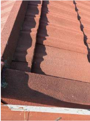
Ref #7.2 - Ridge capping damaged
