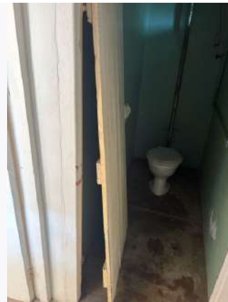
Ref #13.4 - Damaged door
