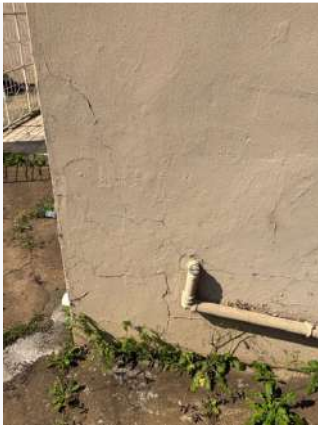
Ref #11.1 - Wall with minor cracks
