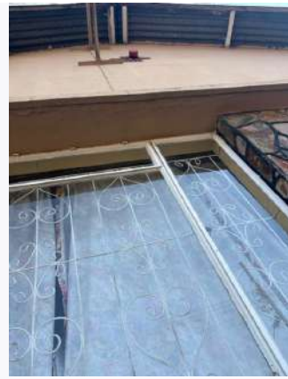
Ref #11.2 - Damaged putty
