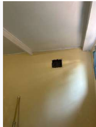
Ref #13.2 - Damaged ceiling
