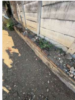
Ref #12.4 - Significant damage to wall
