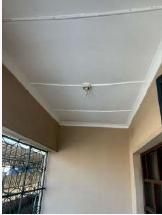
Ref #11.4 - Sagging ceiling
