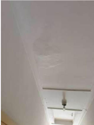
Ref #3.1 - Cracks observed
