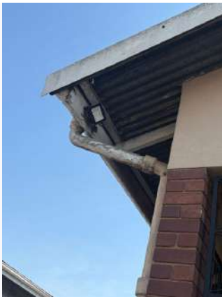
Ref #7.4 - Gutter gutter system infested with debris
