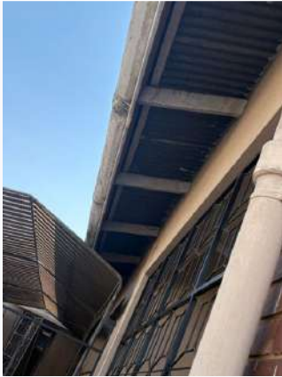
Ref #7.4 - Gutter system infested with debris
