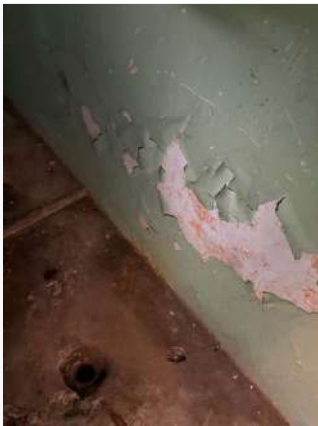
Ref #13.4 - Mold/paint flaking
