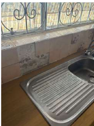
Ref #5.6 - Missing tiles
