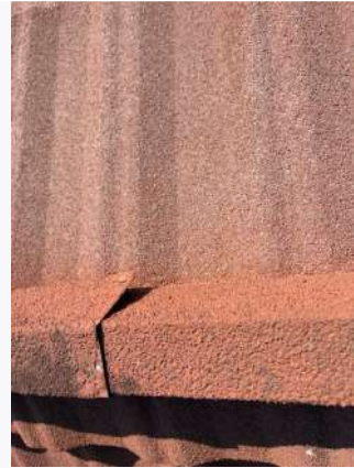
Ref #7.2 - Ridge capping damaged
