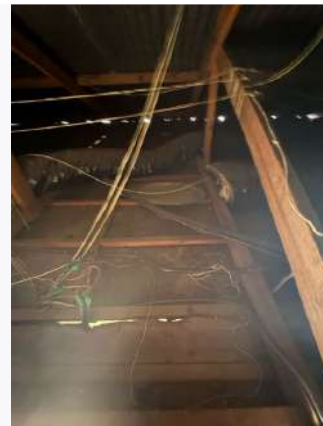
Ref #8.8 - Exposed wiring
