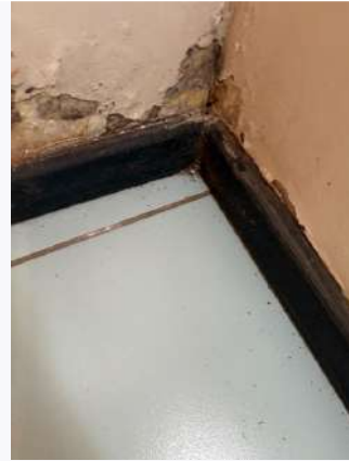
Ref #13.2 - Mold on wall
