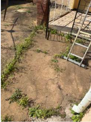
Ref #12.1 - Evidence of water ponding/Ground subsiding
