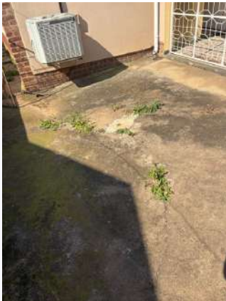
Ref #12.1 - Evidence of water ponding/Ground subsiding
