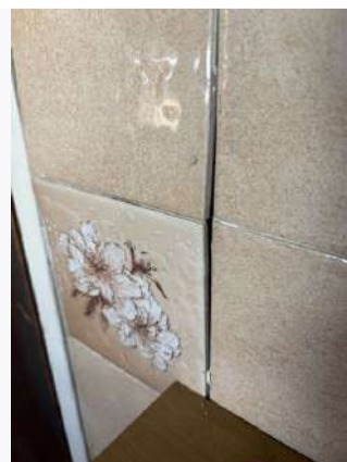
Ref #5.6 - Damaged tiles
