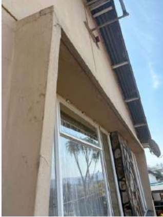
Ref #11.2 - Mold on wall
