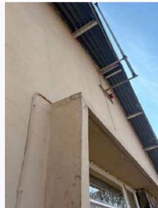
Ref #11.2 - Mold on wall
