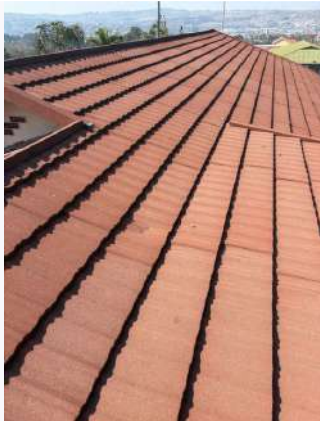
Ref #7.1 - Misaligned /damaged tiles
