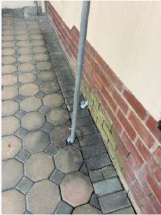
Ref #12.3 - Paving subsided
