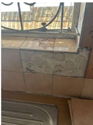
Ref #5.2 - Significant damage to cupboards
