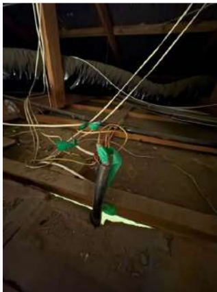
Ref #8.8 - Exposed wiring
