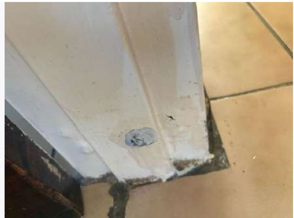
Ref #3.4 - Door frame corroded
