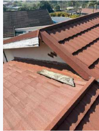
Ref #7.5 - Damaged fascia
