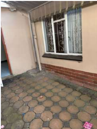
Ref #12.3 - Paving subsided
