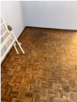
Ref #3.3 - Bedroom 1 floors with wood damage
