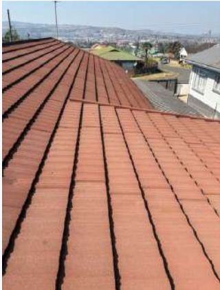
Ref #7.1 - Misaligned /damaged tiles
