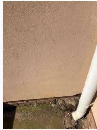
Ref #7.4 - Gutter discharging on unprotected grounds
