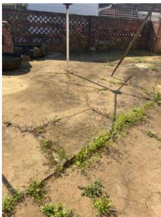
Ref #12.1 - Evidence of water ponding/Ground subsiding
