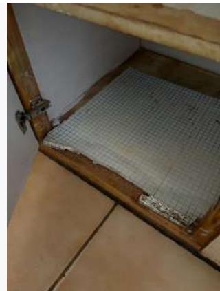
Ref #5.2 - Significant damage to cupboards
