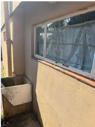
Ref #11.1 - Wall with minor cracks
