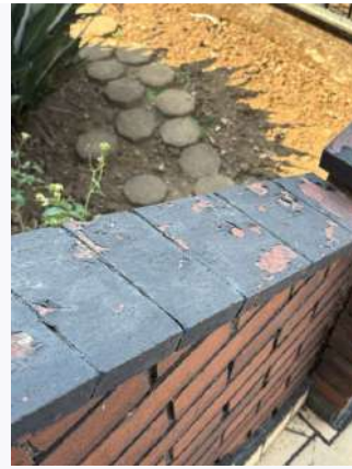
Ref #11.5 - Damaged capping
