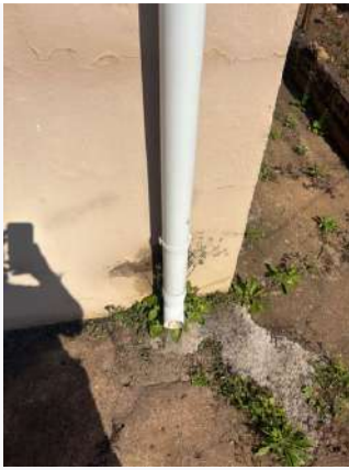
Ref #7.4 - Gutter discharging on unprotected grounds
