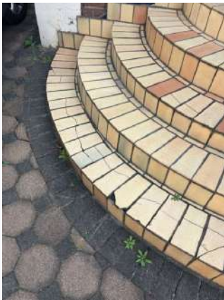
Ref #11.3 - Damaged tiles
