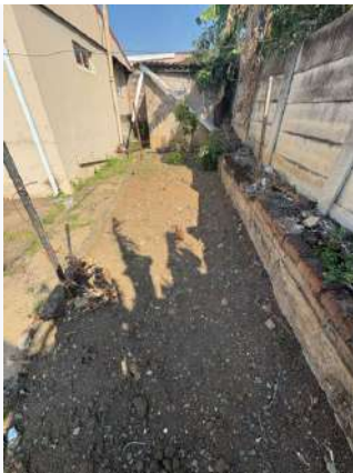
Ref #12.4 - Significant damage to wall
