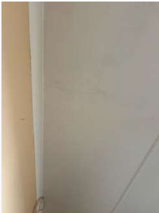
Ref #5.7 - Cracks on ceiling
