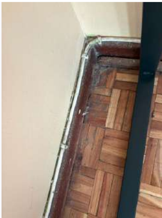
Ref #3.3 - Bedroom 3 floor with wood damage
