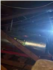
Ref #9 - Geyser with tank
