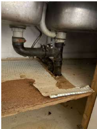
Ref #5.2 - Significant damage to cupboards
