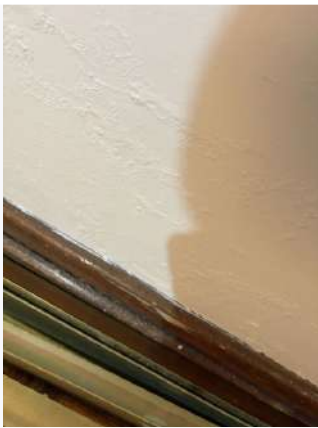
Ref #3.2 - Mold on walls
