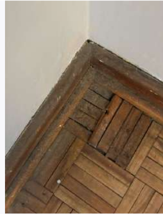
Ref #3.3 - Bedroom 1 floors with wood damage
