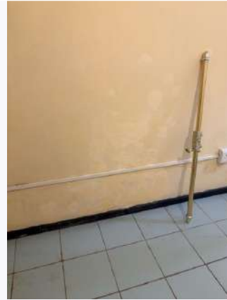
Ref #13.2 - Mold on wall
