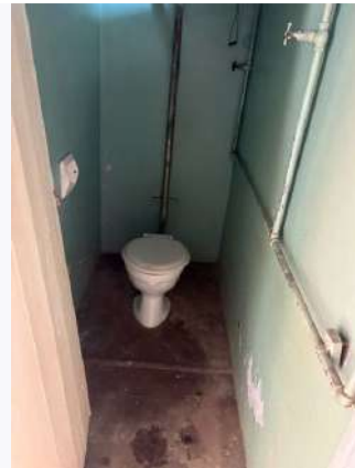
Ref #13.4 - Mold/paint flaking
