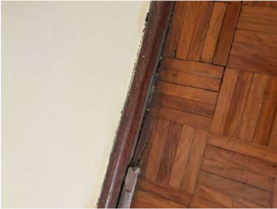
Ref #3.3 - Lounge floor with wood damage
