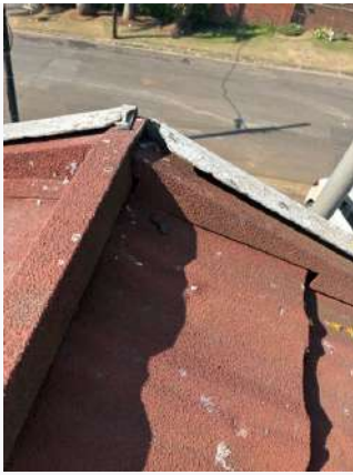
Ref #7.5 - Damaged fascia
