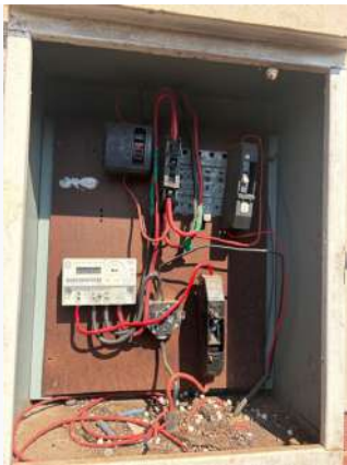
Ref #10.2 - Meter box
