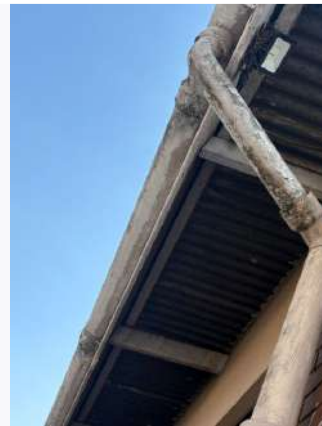
Ref #7.4 - Gutter gutter system infested with debris
