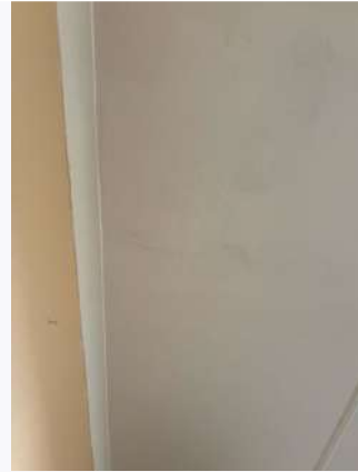
Ref #5.7 - Cracks on ceiling
