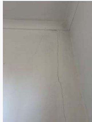
Ref #13.4 - Cracks in walls
