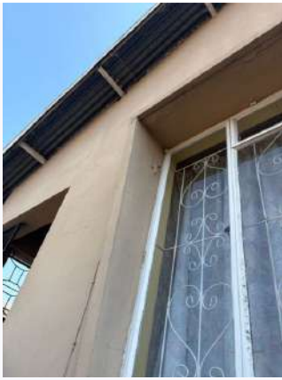
Ref #11.2 - Damaged putty
