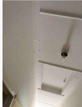
Ref #3.1 - Cracks observed
