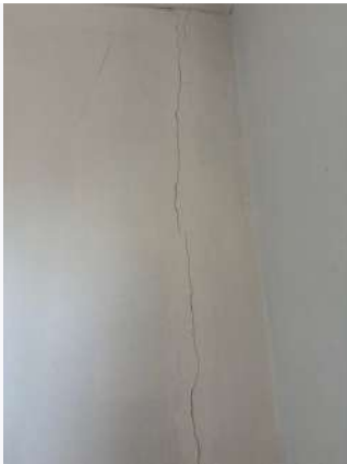
Ref #13.4 - Cracks in walls
