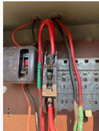
Ref #10.2 - Meter box
