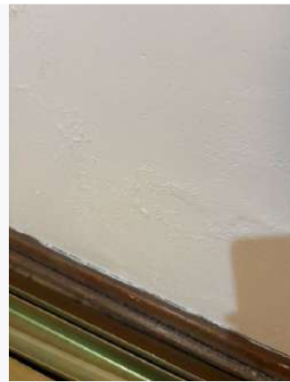
Ref #3.2 - Mold on walls
