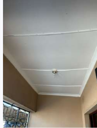
Ref #11.4 - Sagging ceiling
