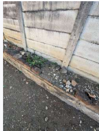
Ref #12.5 - Damage to garden wall
