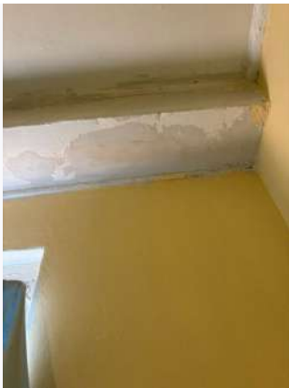
Ref #13.2 - Damaged ceiling
