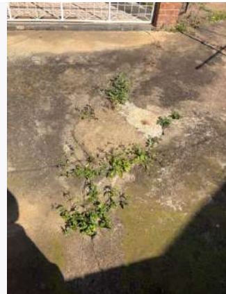
Ref #12.1 - Evidence of water ponding/Ground subsiding
