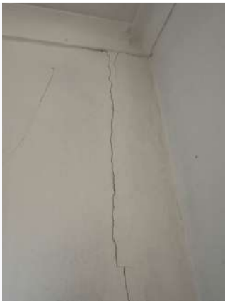
Ref #13.4 - Cracks in walls
