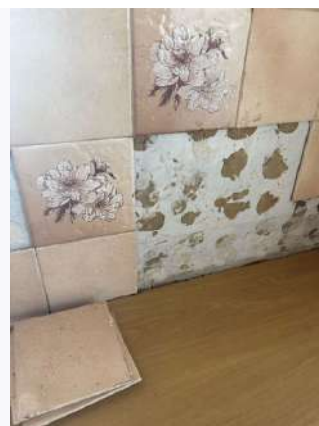
Ref #5.6 - Missing tiles
