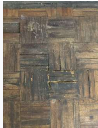
Ref #3.3 - Bedroom 1 floors with wood damage
