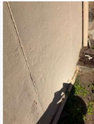
Ref #11.1 - Mold observed on walls
