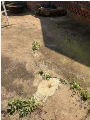
Ref #12.1 - Evidence of water ponding/Ground subsiding
